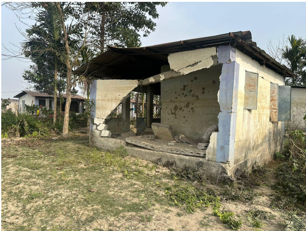
Lots of houses got completely washed away. Many of those which remained are in ruins.
