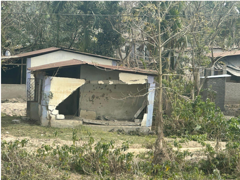
Houses completely shattered after the flood.
